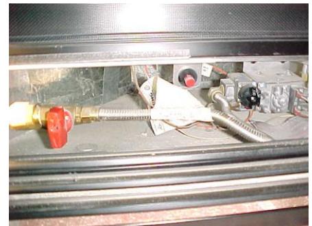
Fireplace gas log controls.
